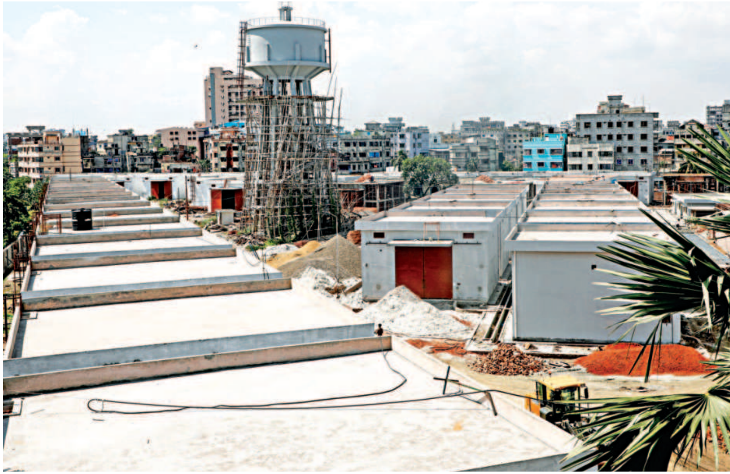
Even after innumerable fire incidents in Old Dhaka, the chemical warehouses and shops are still in the same place. So, it's not a matter of if there will be another fire in the bustling area but when the next incident will occur. That is unless the authorities follow through with their decision to shift the structures to the new site quickly.
