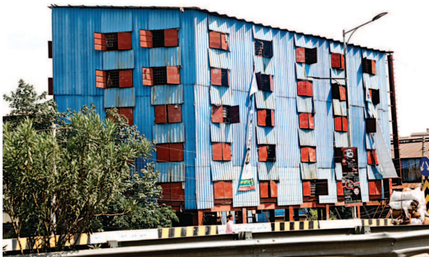
While passing by Postogola area yesterday, this photojournalist came across a rather odd, five-storey tin structure, where labourers of nearby re-rolling mills live. Although it seems to be standing tall for now, it is still doubtful whether this structure even passes the basic fitness check.
