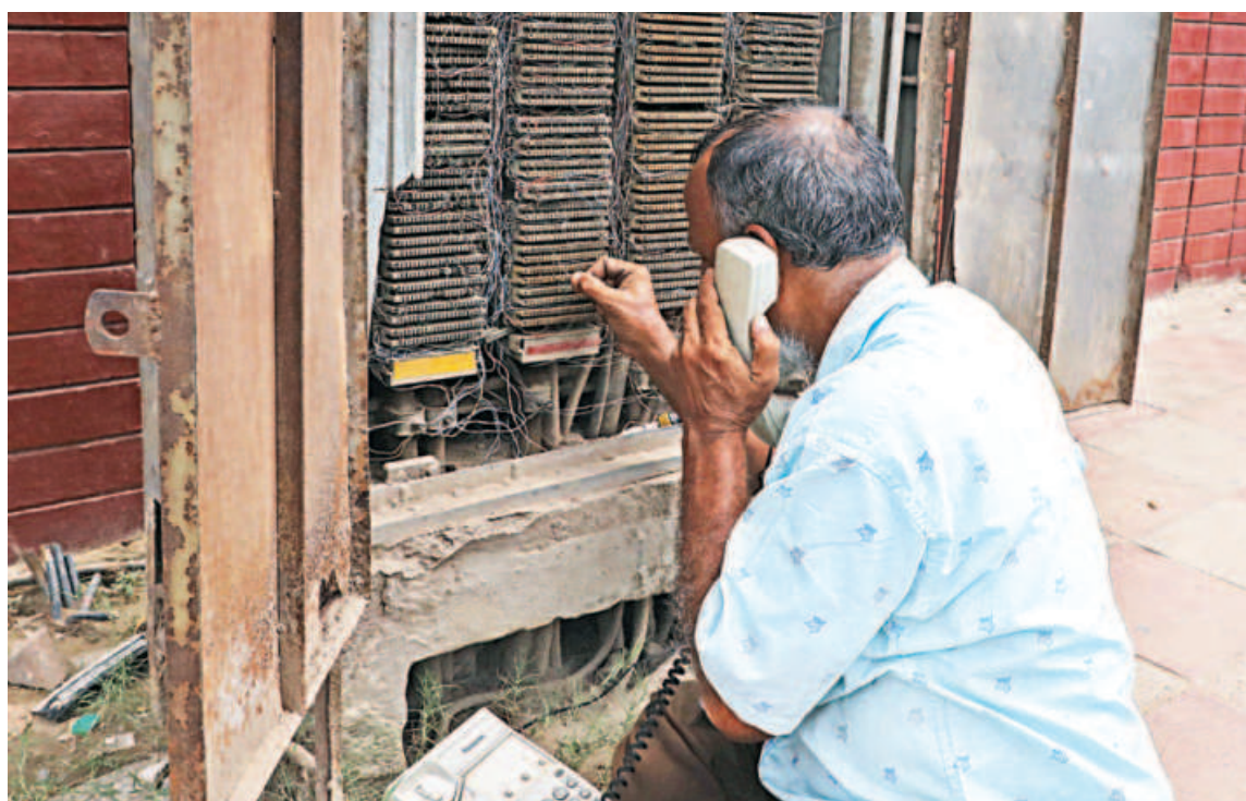
In the age of smartphones and digital devices, landline telephones have almost become obsolete. However, some households and offices that still use such lines have kept the device relevant in the present day. This BTCL employee was spotted opposite BAF Shaheen College in Mohakhali fixing a connection in a grid box. This photo was taken recently.
