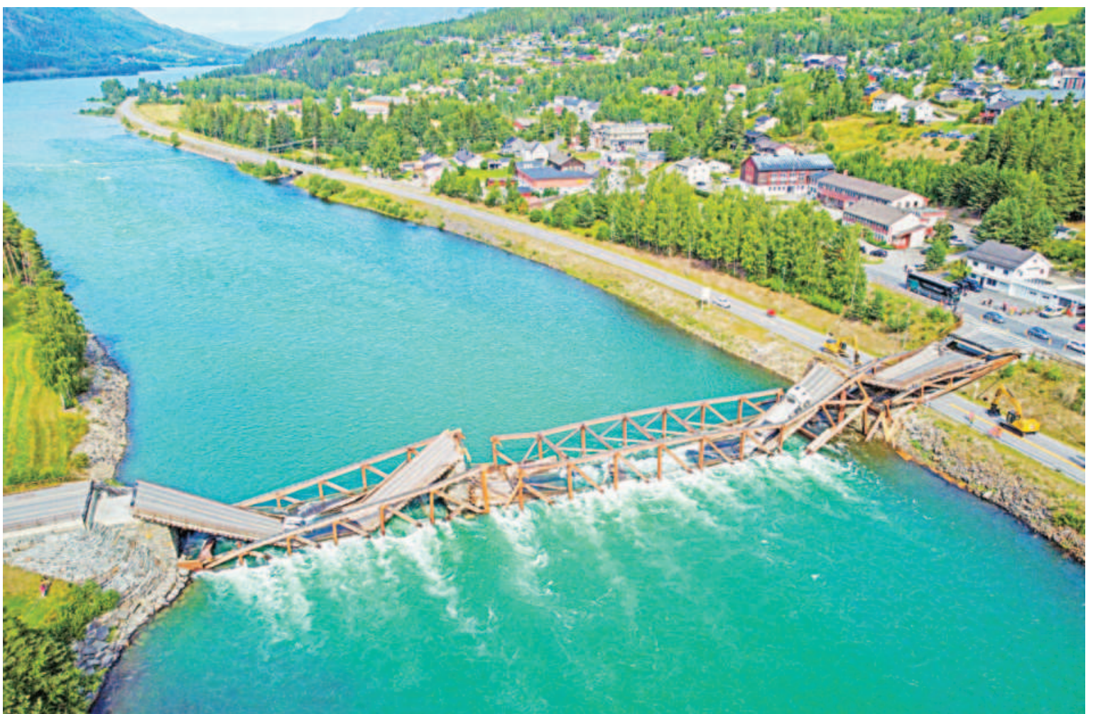
An aerial view shows the collapsed Treffen across the Gudbrandsdalslagen river in the Oyer municipality of southern Norway, yesterday, after it collapsed into the river. Local police report said that a car and truck hurtled into the river.
