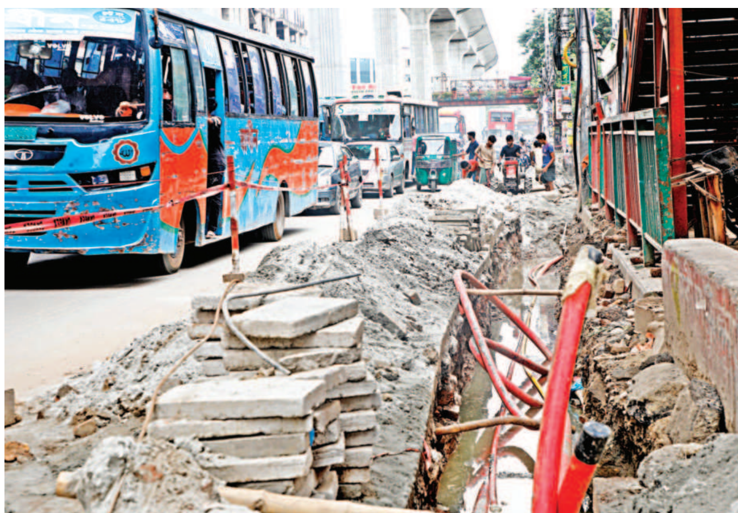
As part of development works, the authorities have dug up a side of the busy Kazi Nazrul Avenue near Karwan Bazar and kept it that way for a while. As work progresses slowly, the biggest sufferers are the commuters, who have to push through gridlock every day while traveling on the road. This photo was taken recently.
