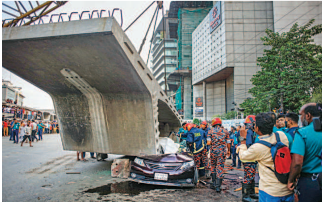
Rescuers search for victims in the mangled remains of a car after a box girder of the under-construction Bus Rapid Transit line-3 fell on it in the capital's Uttara yesterday afternoon. Traffic on the busy road was disrupted for hours after the accident, which claimed five lives. PHOTO: RASHED SHUMON
