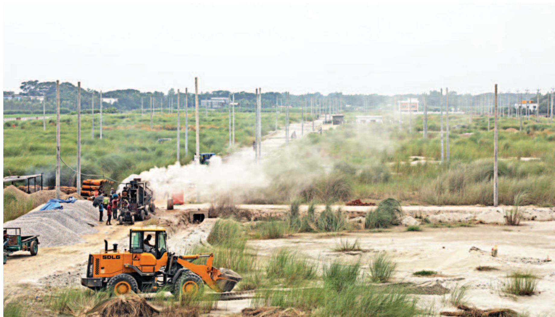
Development work is going on at the country's first industrial park for light engineering and electrical goods sectors in Tongibari upazila of Munshiganj. Initiated in 2016, the estate could not be ready on time owing to land acquisition-related complexity. The photo was taken earlier this month.
