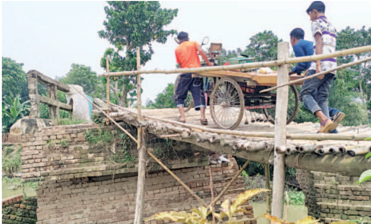
People cross the Panaullah Canal in Nature's Singra upazila as the bridge, which collapsed seven years ago, still lies without repair.
