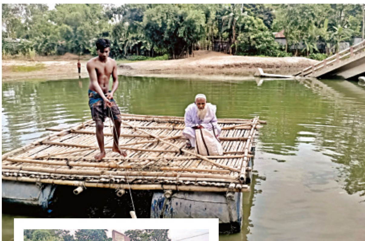
Using a raft, two people crossing the Purba Dhaniram canal in Kurigram's Phulbari on Wednesday. The bridge, inset, built over the canal collapsed on August 22, 2018, before its inauguration. People of seven villages in Barobhita union are affected.
