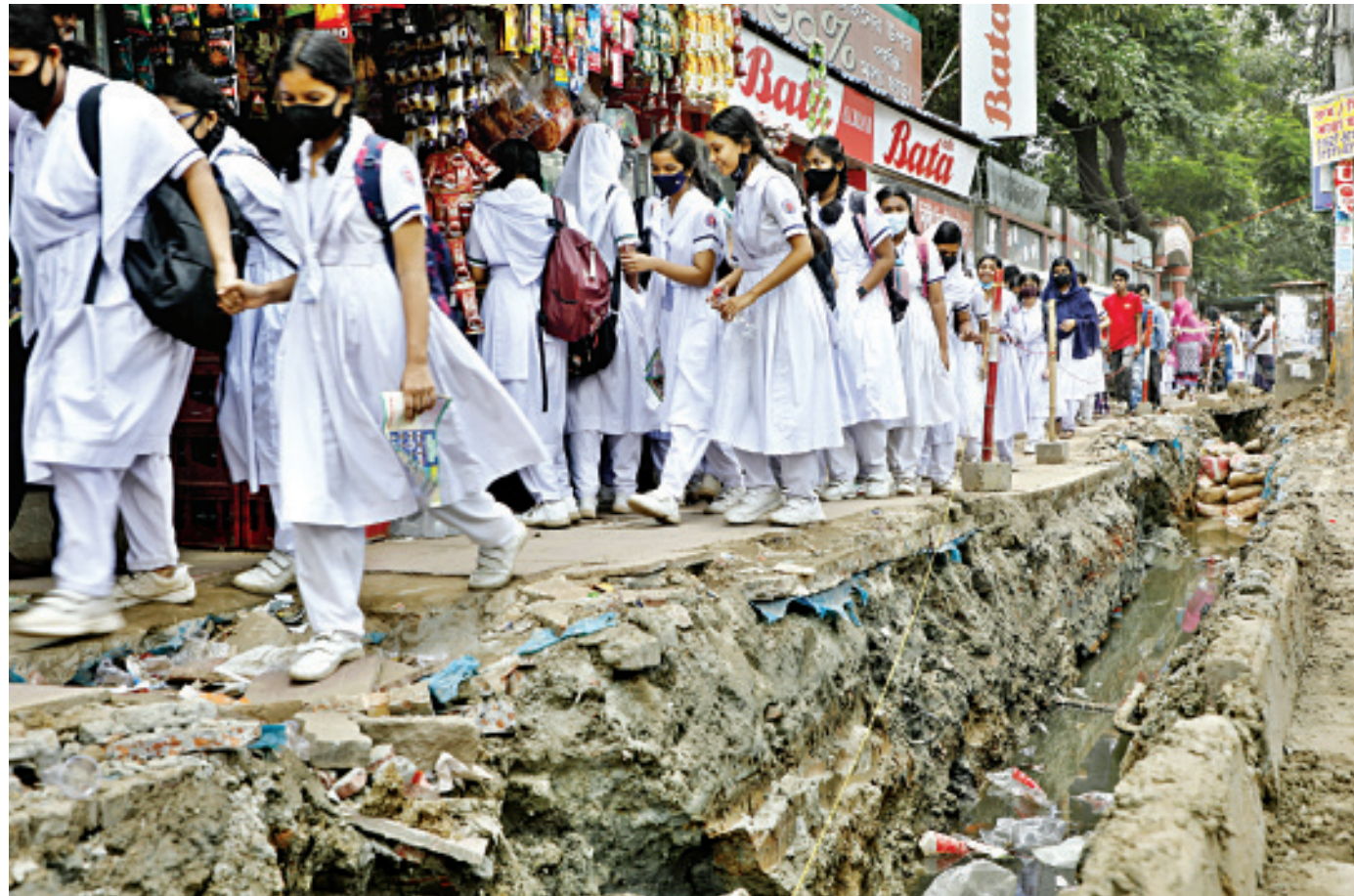
Students walking home on a risky path from Tejgaon Girls' School and College in the capital yesterday. The roads in the area have been dug up to install underground electric lines. Locals said the work has been going on for over a week, causing distress to commuters.
