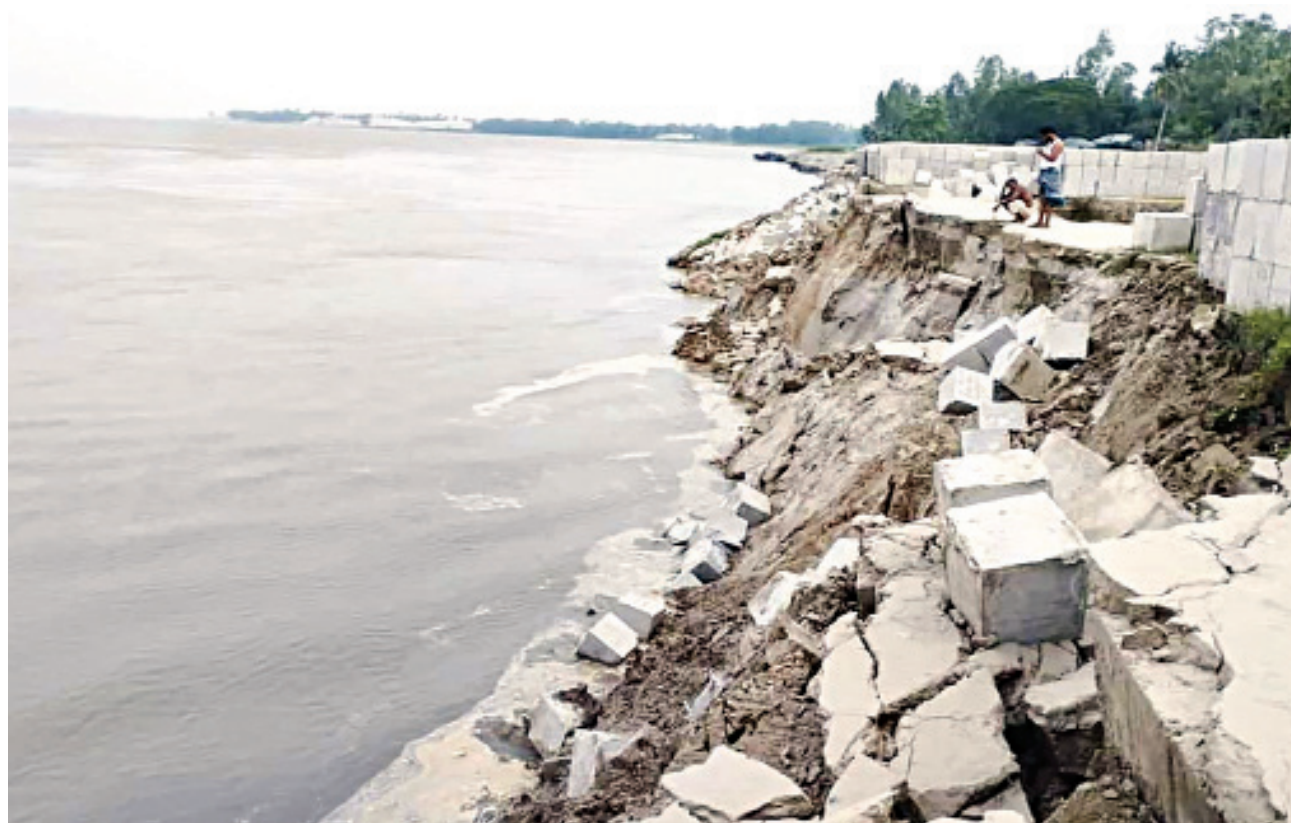
Erosion has hit a 200-metre stretch of the Jamuna riverbank in Sirajganj's Kazipur upazila. The Water Development Board is dumping sand-filled bags in the area to reduce the damages. The photo was taken on Friday.
