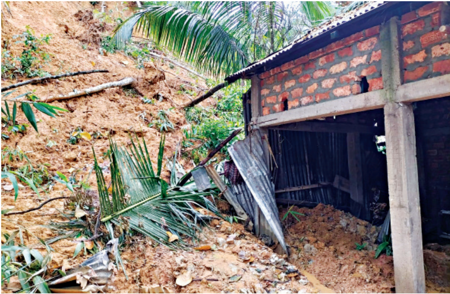
In the aftermath of last month's downpour, 49 families in Moulvibazar's Zuri upazila have lost their homes to a devastating landslide. Many had to move to shelters, while some left the area forever. Locals alleged that although a month had gone by, they are yet to receive any kind of relief or assistance from the government.
