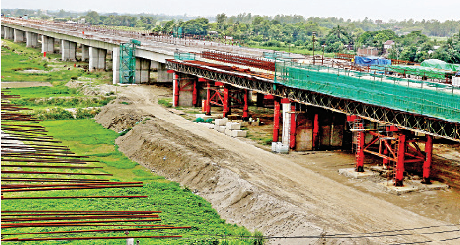
Development work is ongoing at the Padma Bridge Rail Link project in Keraniganj. The government's spending on projects under the annual development programme returned to almost pre-pandemic levels in the previous fiscal year as work resumed following two years of disruption due to Covid-19.
