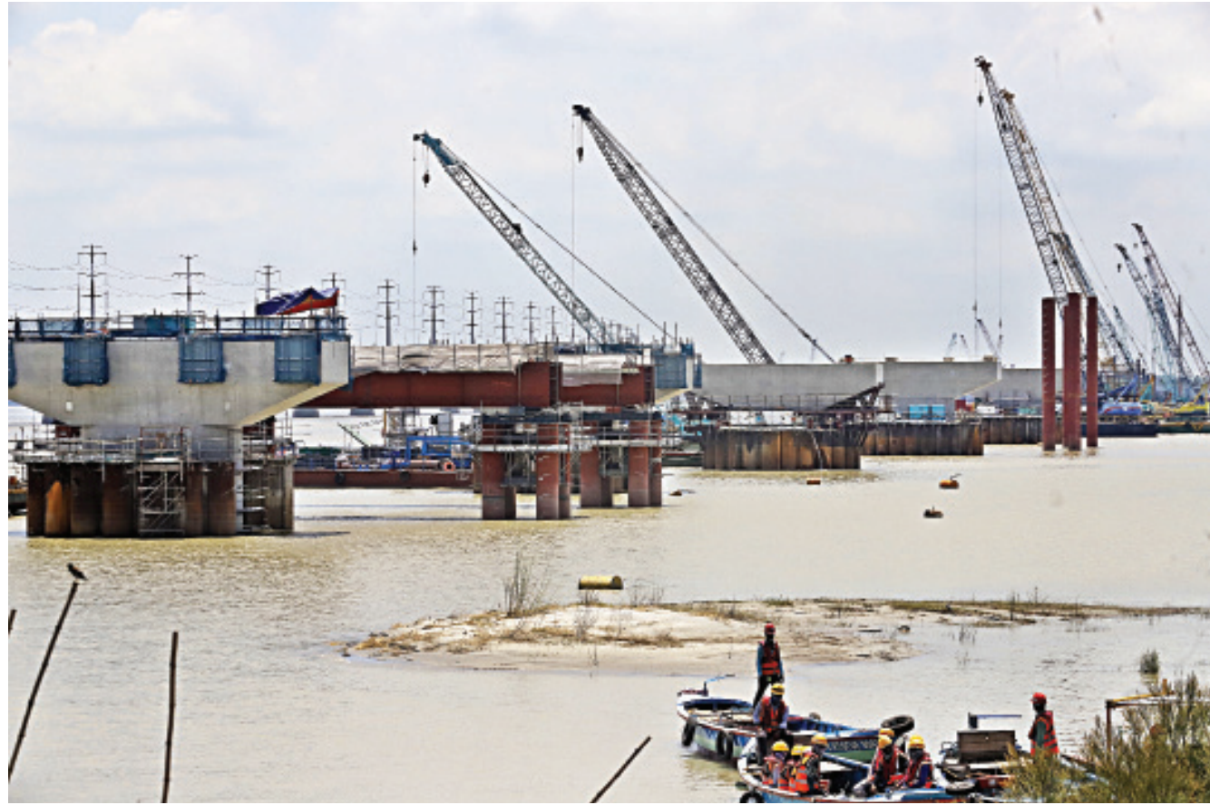
Construction work of Bangabandhu Sheikh Mujib Railway Bridge is in progress over the Jamuna river. The photo was taken recently at the eastern side of the river. The bridge will be a major leap for railroad communication in the country.
