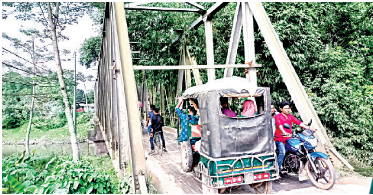
This narrow bridge over the Ratnai river at Kalughat in Lalmonirhat Sadar upazila is a setback for development, depriving people of getting benefits of the newly-built Dharla Bridge. PHOTO: STAR
