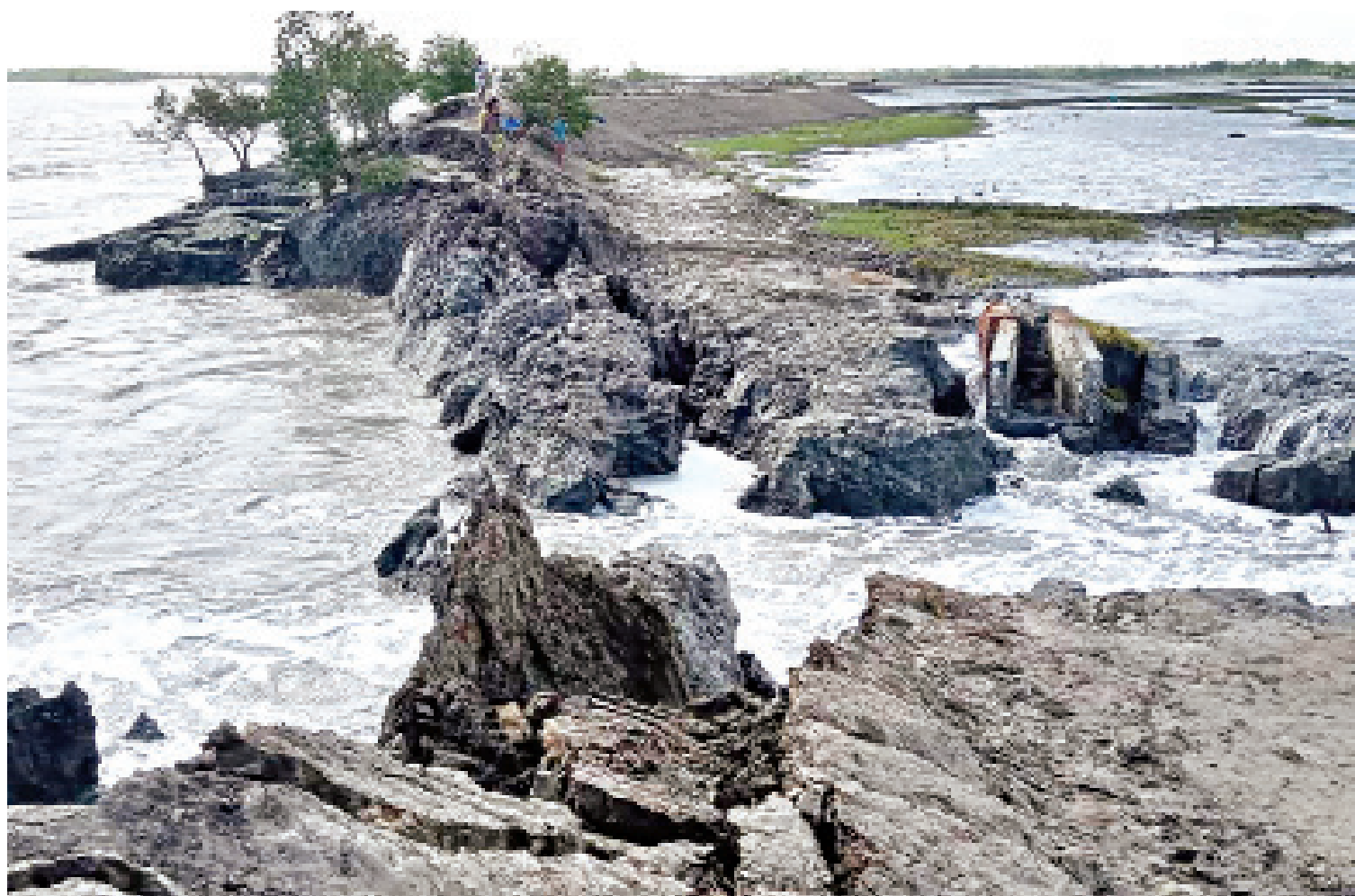
The collapse of the 150-foot embankment at Durgabati point in Kholpetua River left hundreds of people marooned, inundated croplands and washed away shrimp enclosures. Four villages of Satkhira's Shyamnagar upazila have been submerged due to the embankment's collapse.
