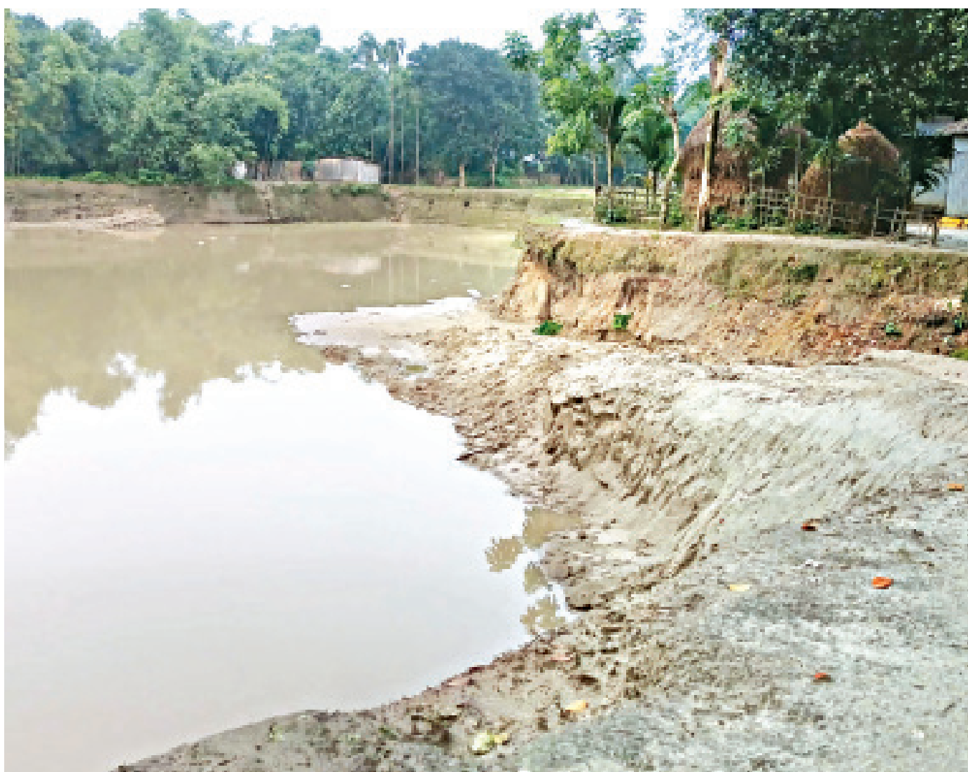
Defying the law, a local influential man has been constructing these shops taking lease of a rural market in Tangail's Ghatail upazila.
