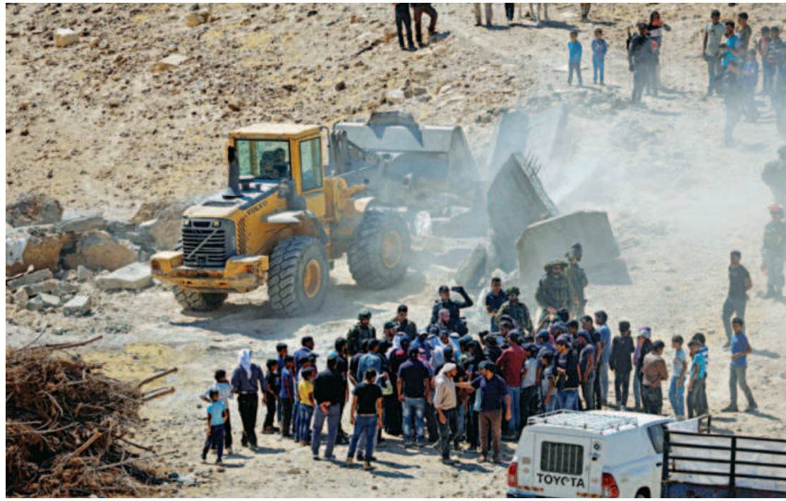
People gather as an Israeli machinery guarded by Israeli forces demolish a Palestinian house in Masafer Yatta, in the Israeli-occupied West Bank yesterday.
