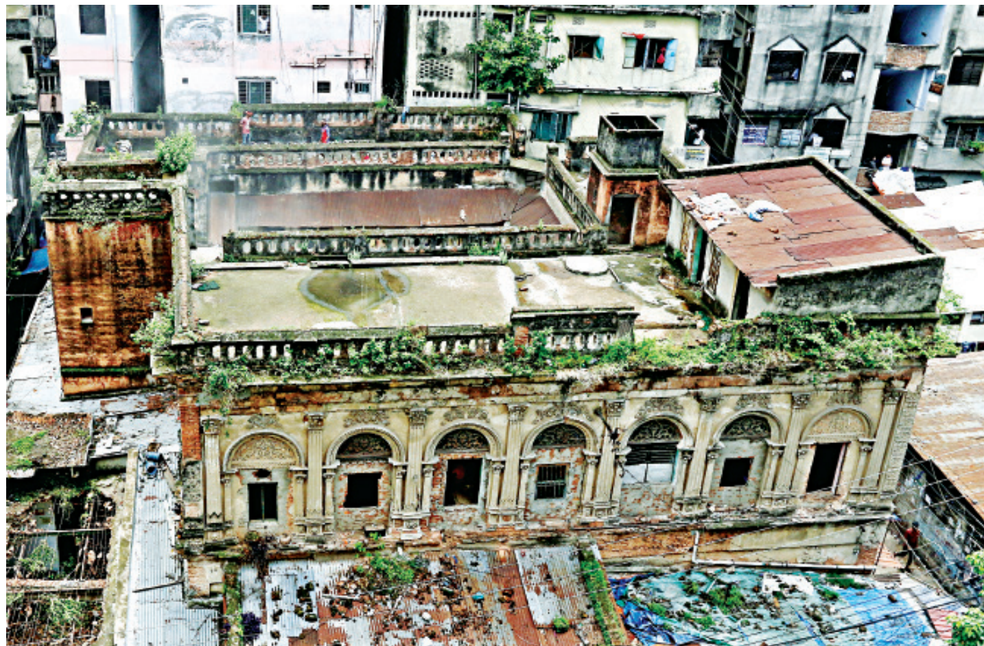
Around 30 to 35 labourers are working to knock down the Neelam Ghar to build a new structure for Dhaka Bar Association. The century-old establishment on the Court Street in Old Dhaka is recognised by conservationists as a rare feat of masonry. The property has been leased out to the association by the deputy commissioner's office. The association is now planning to construct a multi-storey building by demolishing this structure. However, when asked, they claimed that they are only running renovation works on the building. This photo was taken yesterday.
