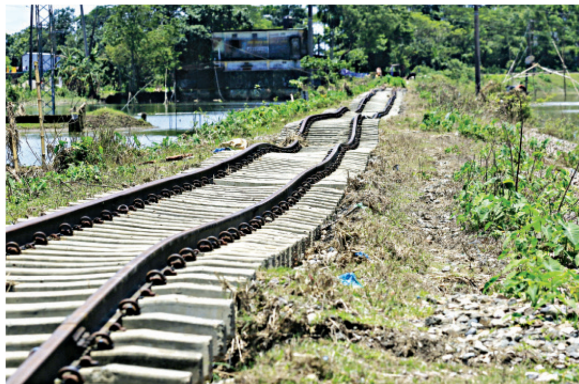
With floodwaters receding in many areas in Sylhet division, a trail of devastation is becoming visible. These rail lines in Chhatak upazila of Sunamganj, which had been under water for days, appear to be warped as the gravel underneath got washed away.
