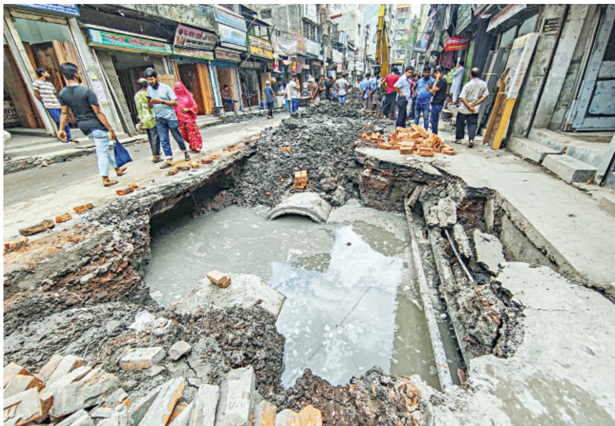
This and several other large holes dug in the middle of the road in Nayabazar over two months ago by Dhaka South City Corporation have been the cause of frequent mishaps and a constant inconvenience for the locals. PHOTO: RASHED SHUMON
