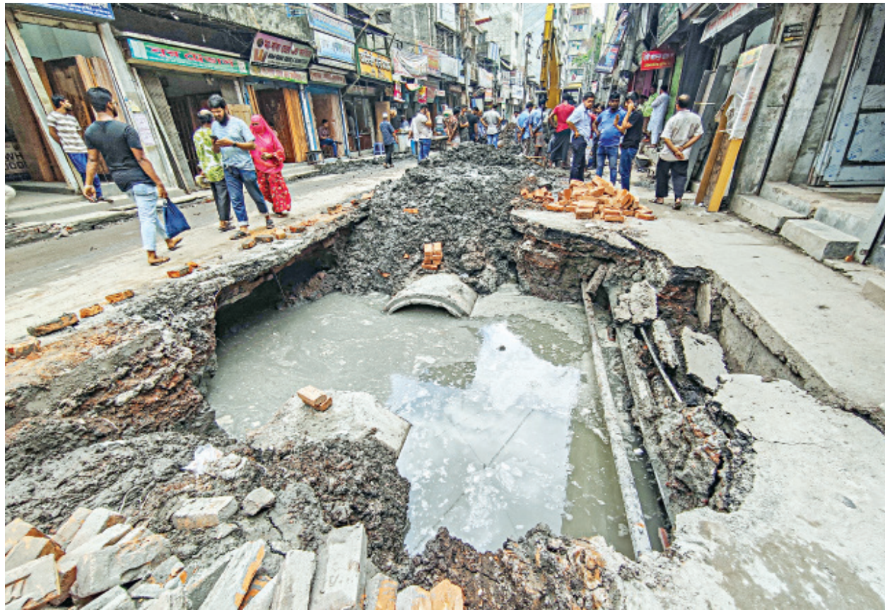
This and several other large holes dug in the middle of the road in Nayabazar over two months ago by Dhaka South City Corporation have been the cause of frequent mishaps and a constant inconvenience for the locals. PHOTO: RASHED SHUMON
