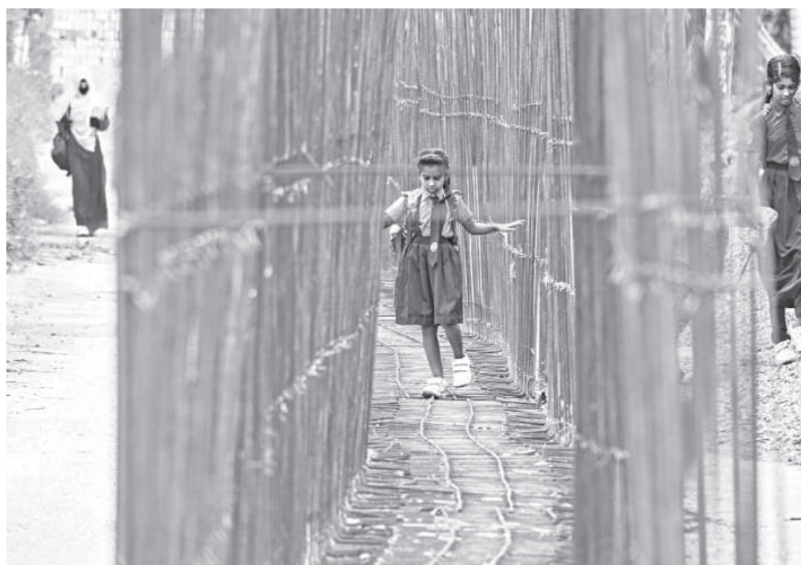
For over a month now, the authorities have left a rod structure meant for the construction of a drain right in the middle of Sonadanga-Notun Rasta road. For this, school children from surrounding areas have to face much difficulty to get across. This photo was taken from Boyra area in Khulna recently.
