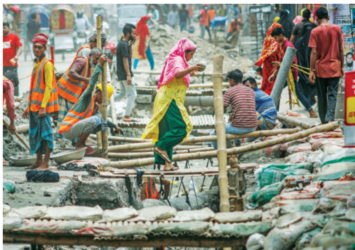
A large part of the main road at Dhaka Udyan was dug up by authorities over two months ago to install an underground cable line. Makeshift bamboo planks have been set up, using which pedestrians have to cross the area, putting themselves at risk of accidents. This photo was taken from Mohammadpur yesterday.
