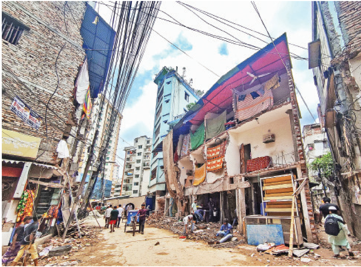
Buildings remain half destroyed after City Corporation authorities carried out eviction drives against illegal establishments -- including residential buildings, shops and factories -- at the Kathalbagan Box culvert road a month and half ago. People have begun living in the partly-demolished structures, which might result in tragic accidents. The photo was taken yesterday.
