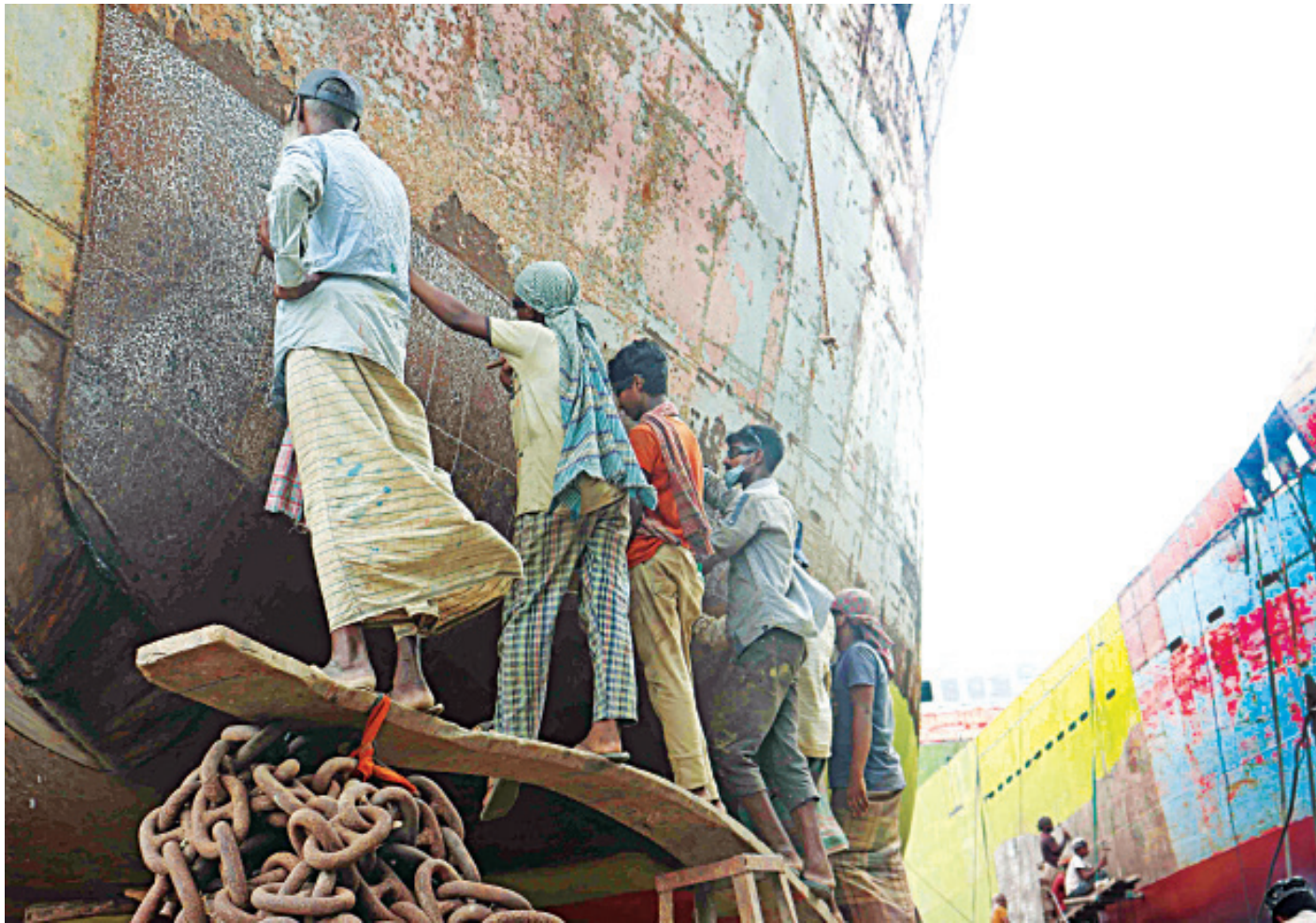
Ship repairs and refurbishment are heavily dependent on manual labour, requiring five categories of workers, including welders, grinding and fitting specialists and painters. Hundreds of people make a living working in rudimentary dockyards along the banks of the Sandhya river in Pirojpur's Nesarabad upazila. Around 10 types of vessels are also built here, from iron trawlers to cargo boats, varying in length from 30 feet to 250 feet. The photo was taken last week.
