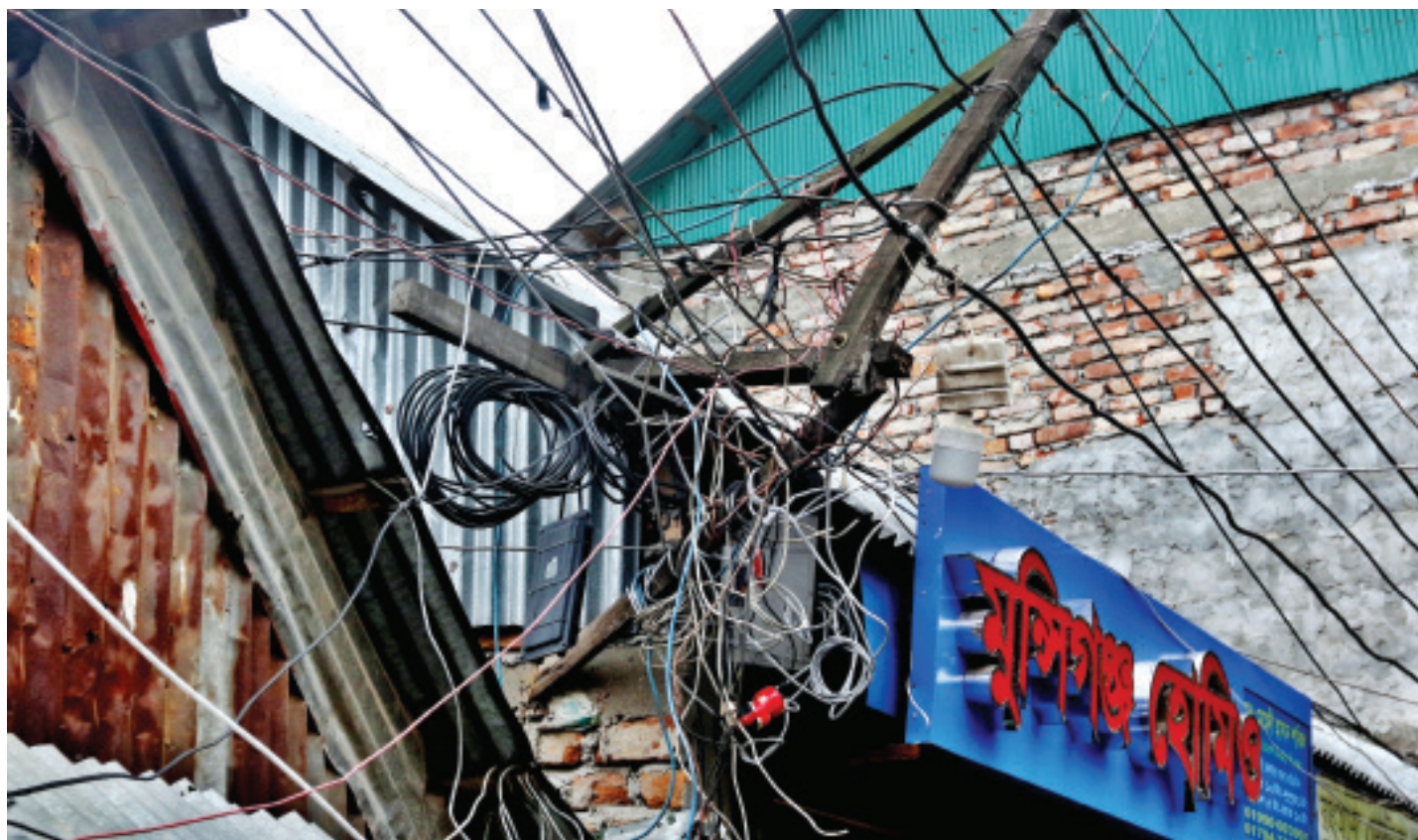
A tangle of electrical cables next to a shed in the capital's Korail slum. Hundreds of these wires snake through the slum, posing fire risks as most of the connections are illegal and therefore not installed following the proper procedures. The photo was taken on Thursday.
