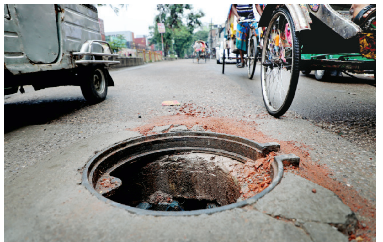
Right in the middle of the main road in front of Kamalapur Railway Station, speedy vehicles were seen going past a gaping manhole. Despite days going by since the cover was spotted missing, authorities are yet to fix a lid on it. This in itself poses risks of accidents but during the ongoing monsoon, the chances of unfortunate events occurring grow manifold. This photo was taken yesterday.
