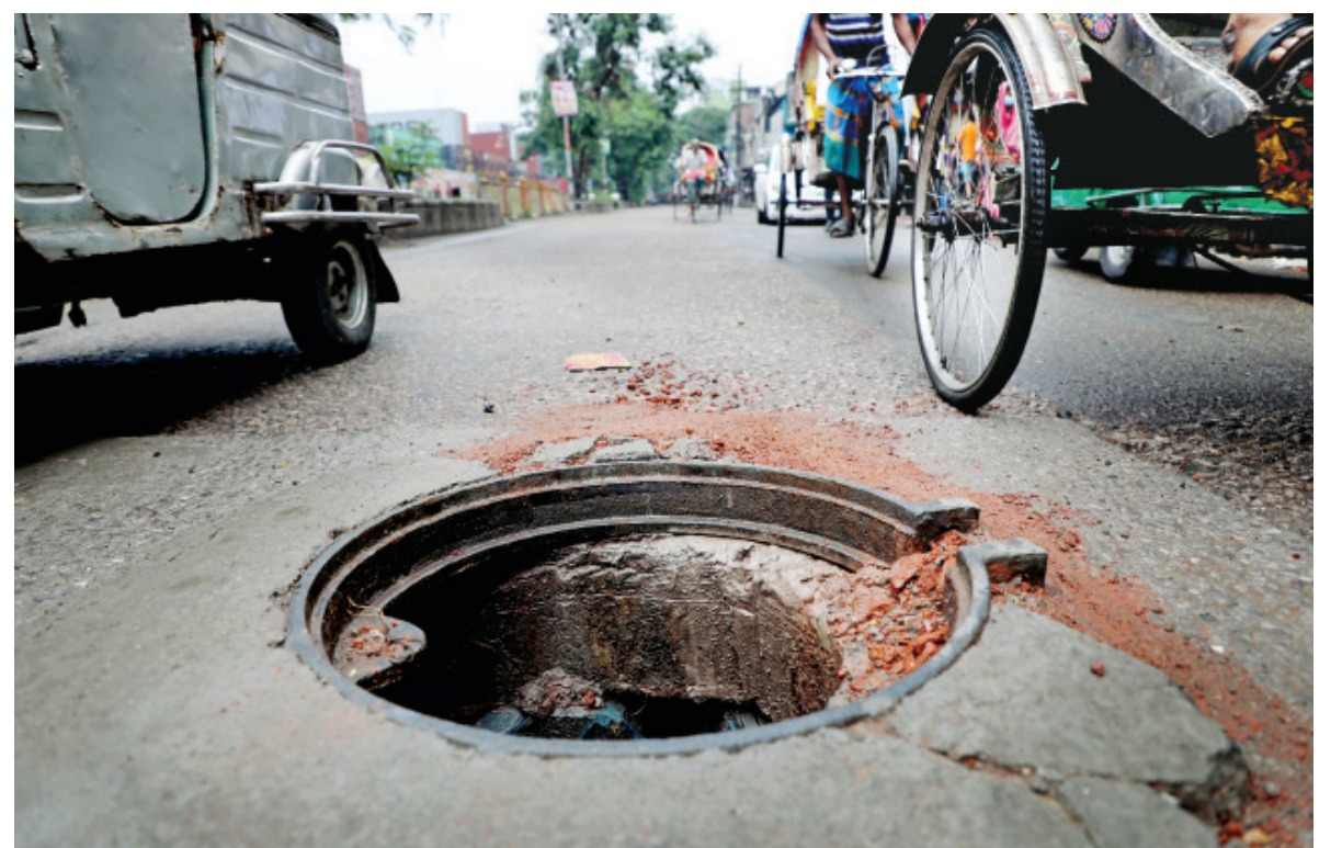
Right in the middle of the main road in front of Kamalapur Railway Station, speedy vehicles were seen going past a gaping manhole. Despite days going by since the cover was spotted missing, authorities are yet to fix a lid on it. This in itself poses risks of accidents but during the ongoing monsoon, the chances of unfortunate events occurring grow manifold. This photo was taken yesterday.
