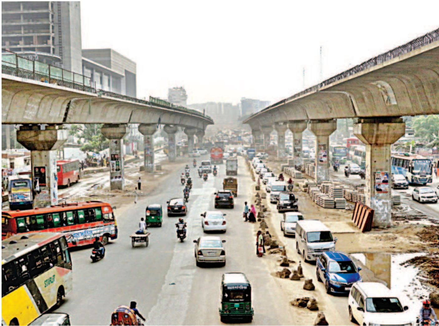
Amidst the bustle of vehicles on the busy Kurmitola Road, construction work of Dhaka Elevated Expressway and the metro rail can be seen at the same time, as progress steadily continues. This photo was taken yesterday.
