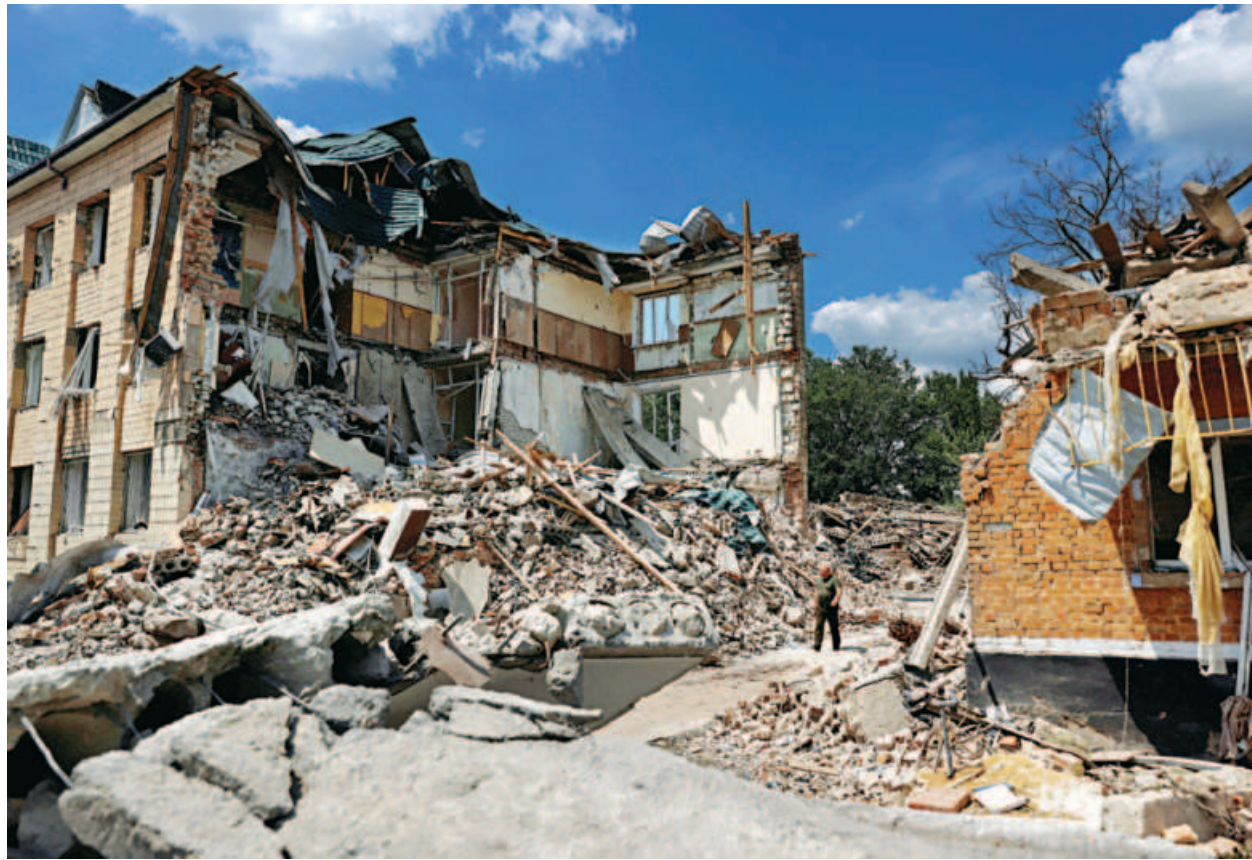
A destroyed city administration building in Bashtanka, Mykolaiv region, as Russia's attack on Ukraine continues. The photo was taken Thursday. PHOTO: REUTERS
