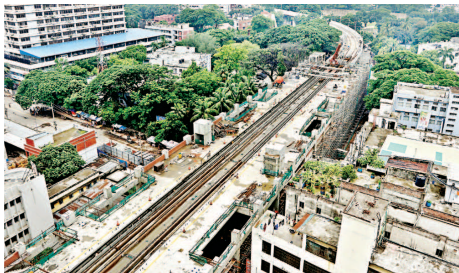
A metro rail station being built in front of the Jatiya Press Club on the capital's Tophkana Road. Work is also underway to lay tracks on this section of the Mass Rapid Transit Line-6. The photo was taken yesterday.
