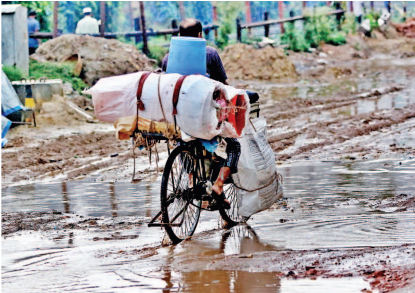
Owing to the construction work of Dhaka Elevated Expressway, the road near Tejgaon rail-crossing has been in a terrible condition. Even after a drizzle, muddy puddles cover the entirety of the path, as many parts of the road have been excavated. As a result, it is now a daunting task to cross this road. This photo was taken yesterday.
