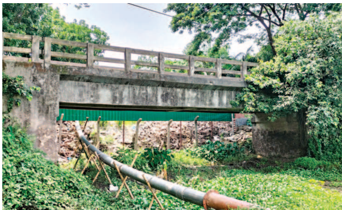
Hundreds of farmers at Purangram village in Manikganj's Ghior upazila are being affected after a company illegally erected structures on an irrigation canal beside Manikganj-Tangail road. The photo was taken recently.
