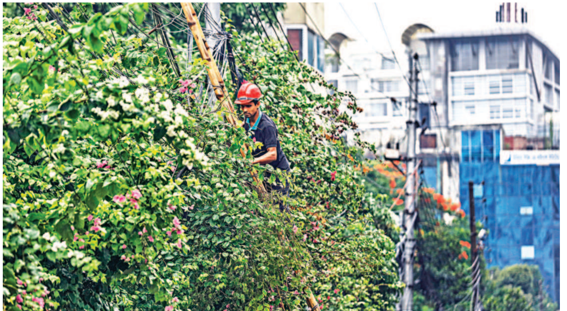
On the rare occasions when nature and greeneries become obstacles to modern amenities in the urban spaces, human intervention becomes inevitable. Yesterday, this electrician was seen cutting the expanded tree branches and leaves that fell on the high-voltage electric wires to prevent any unwanted accident. The photo was taken in Paribagh.
