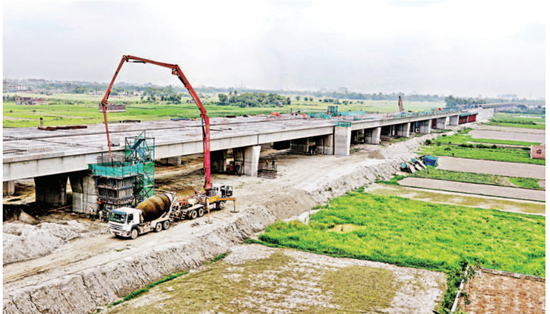
Work for the Padma Bridge Rail Link Project is going on in full swing in South Keraniganj, where an elevated station is being built. Under the Tk 39,246.80 crore project, a 169-kilometre rail route would be built from the capital, through the Padma bridge, to Jashore. The photo was taken yesterday.
