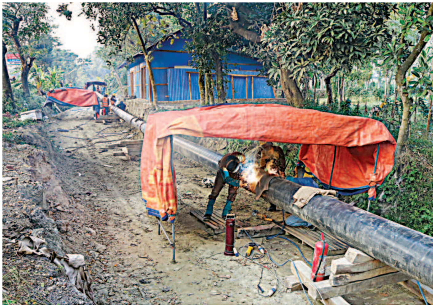
Workers are seen welding together two sections of the 250-kilometre fuel pipeline between Chattogram and Dhaka. Being implemented at a cost of about Tk 3,172 crore, the project is scheduled to be complete by this December. The photo was taken in Sitakunda upazila of Chattogram recently.
