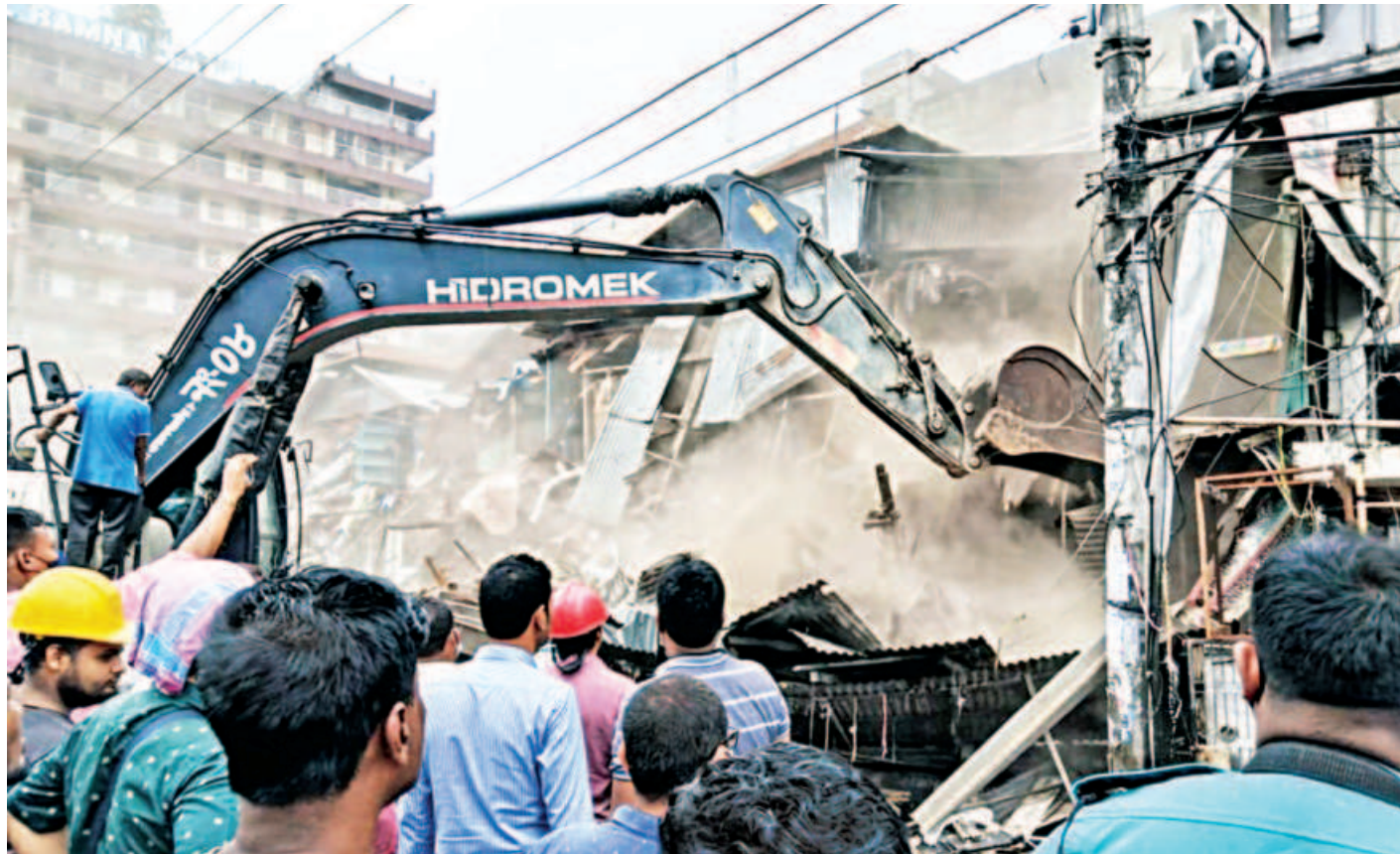
An excavator demolishing illegal structures of the hawkers' market on Bangabandhu Avenue yesterday. Around 100 such structures were knocked down by the Dhaka South City Corporation to free the space from the illegal occupants.
