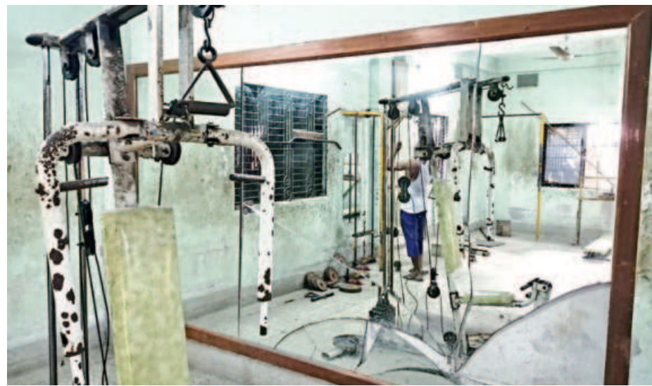
At Sutrapur Modern Gymnasium, the equipment are covered in rust and the plaster is coming off the walls. Those who are regulars at the gym said the situation has not improved in years.
