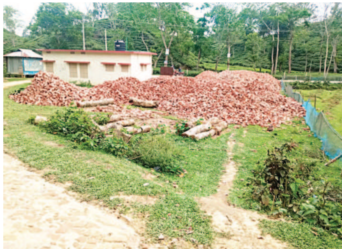
The road through Lathitila Protected Forest was being constructed under the initiative of LGED, without the forest department's approval. The construction is currently suspended after forest officials' intervention.
