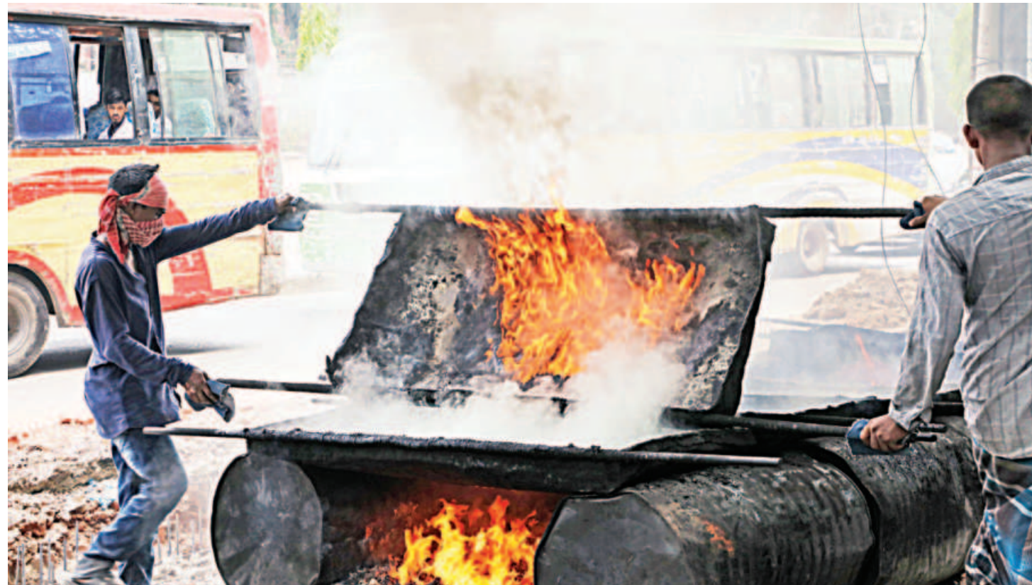
With no safety gear on and no masks to protect them from the fumes, workers are busy melting asphalt for the city's road construction work in an extremely hazardous environment. This photo was taken at the capital's Agargaon yesterday.
