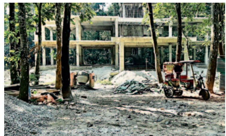
The construction of a two-storey rest house is underway on another land adjacent to where the artificial lake is supposed to be dug.
