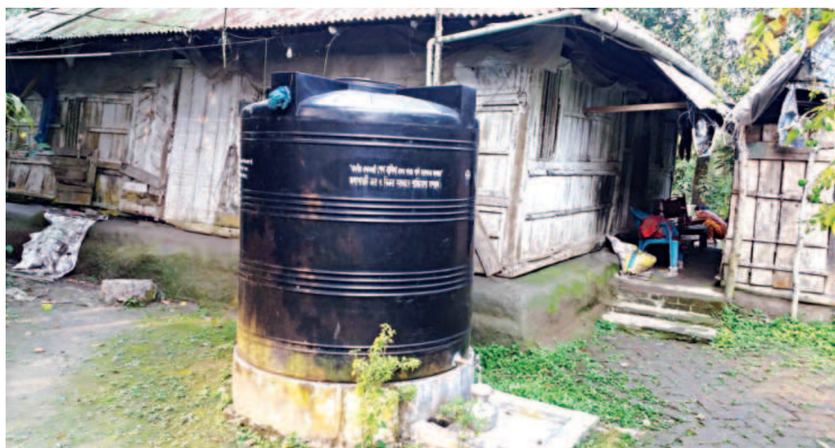
Rainwater harvesting tanks have been set up at homesteads of the people living in the coastal areas, thanks to DPHE. The tanks are likely to come as a respite for the people who suffer from acute freshwater crisis in summer. PHOTO: STAR
