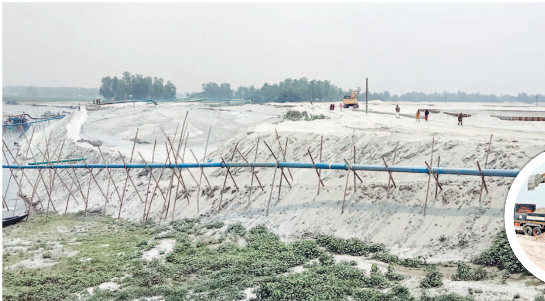
Land development nearing completion by the Jamuna river for an industrial park of the Bangladesh Small and Cottage Industries Corporation in Sirajganj. However, only five out of 17 categories of works have been completed, with the authorities set to seek a one-year extension of the completion deadline. The photo was taken yesterday.
