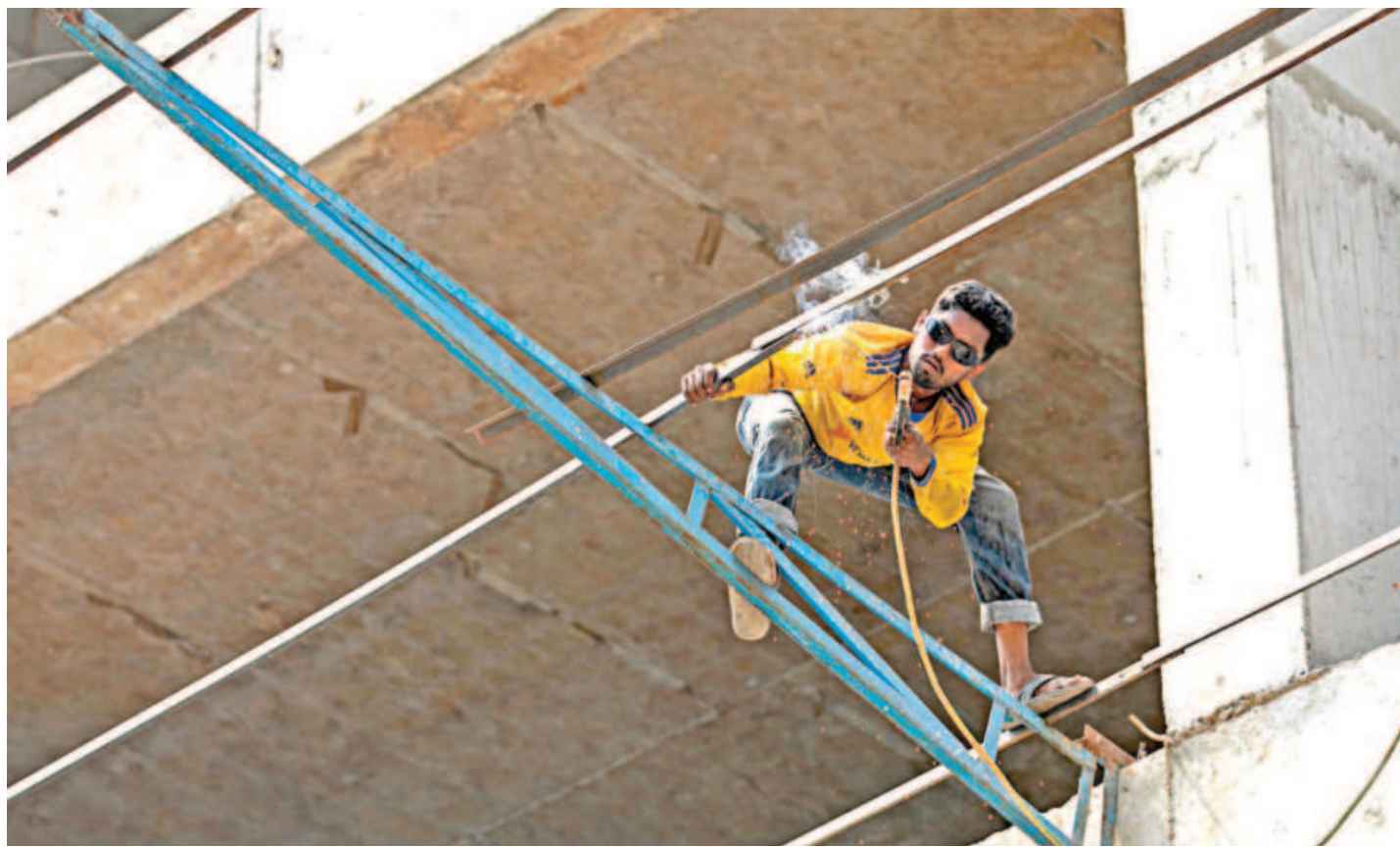
With no safety gear in sight, a man stands precariously on a flimsy metal beam to weld construction material of a building. Such sights are not a rarity, as these workers regularly put their lives on the line while authorities turn a blind eye. The photo was taken yesterday in port city's Prabartak area.
