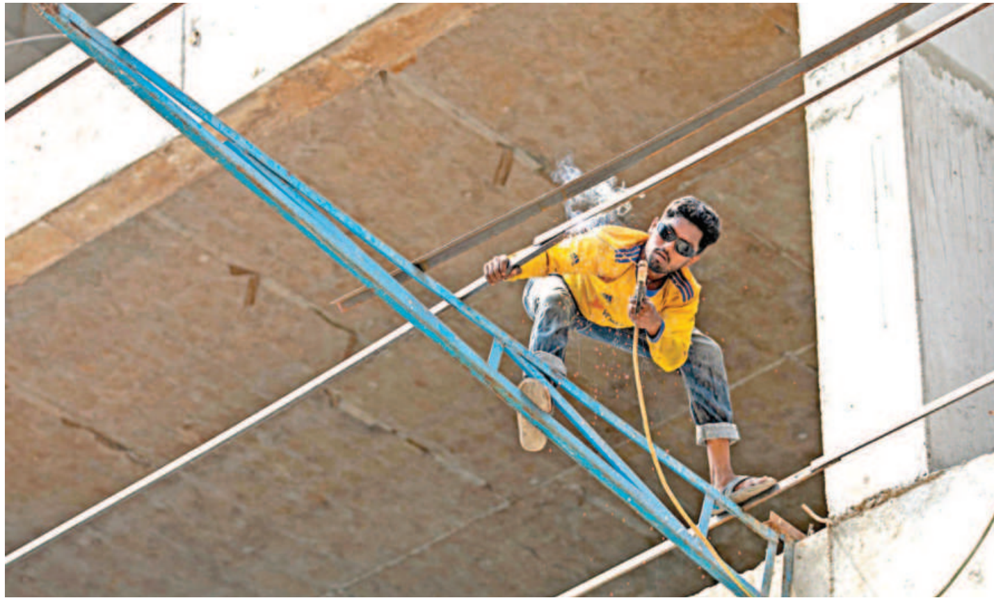
With no safety gear in sight, a man stands precariously on a flimsy metal beam to weld construction material of a building. Such sights are not a rarity, as these workers regularly put their lives on the line while authorities turn a blind eye. The photo was taken yesterday from port city's Prabartak area.
