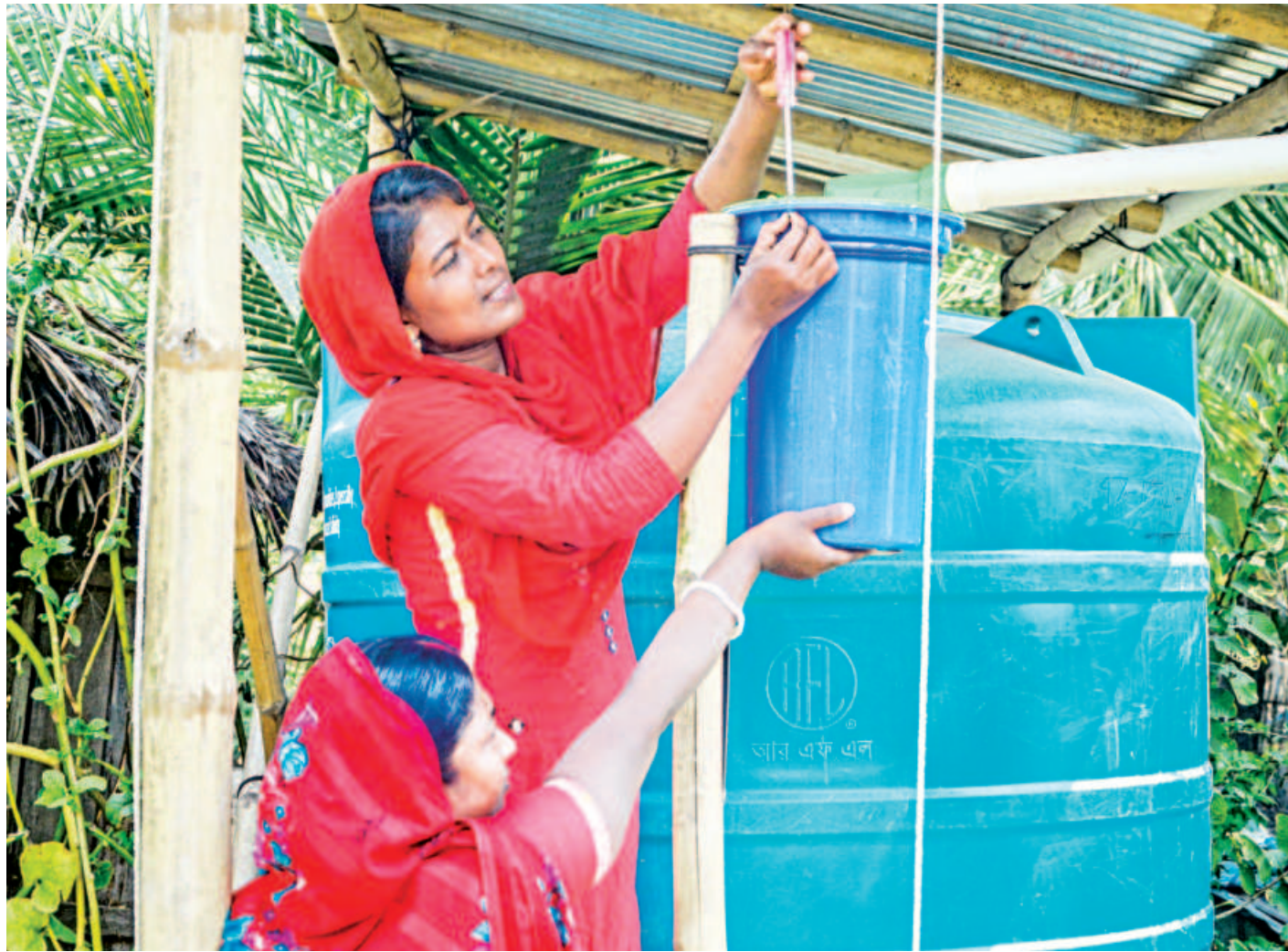
Raushan Ara Akhter (32), locally known as "Paani Apa", has been working as a one-woman army in the battle against the water crisis in Gunari village of Khulna's Dakop upazila. She goes door-to-door, fixing the water tank pipelines in every house to install rainwater harvesting systems and clean the filter.
