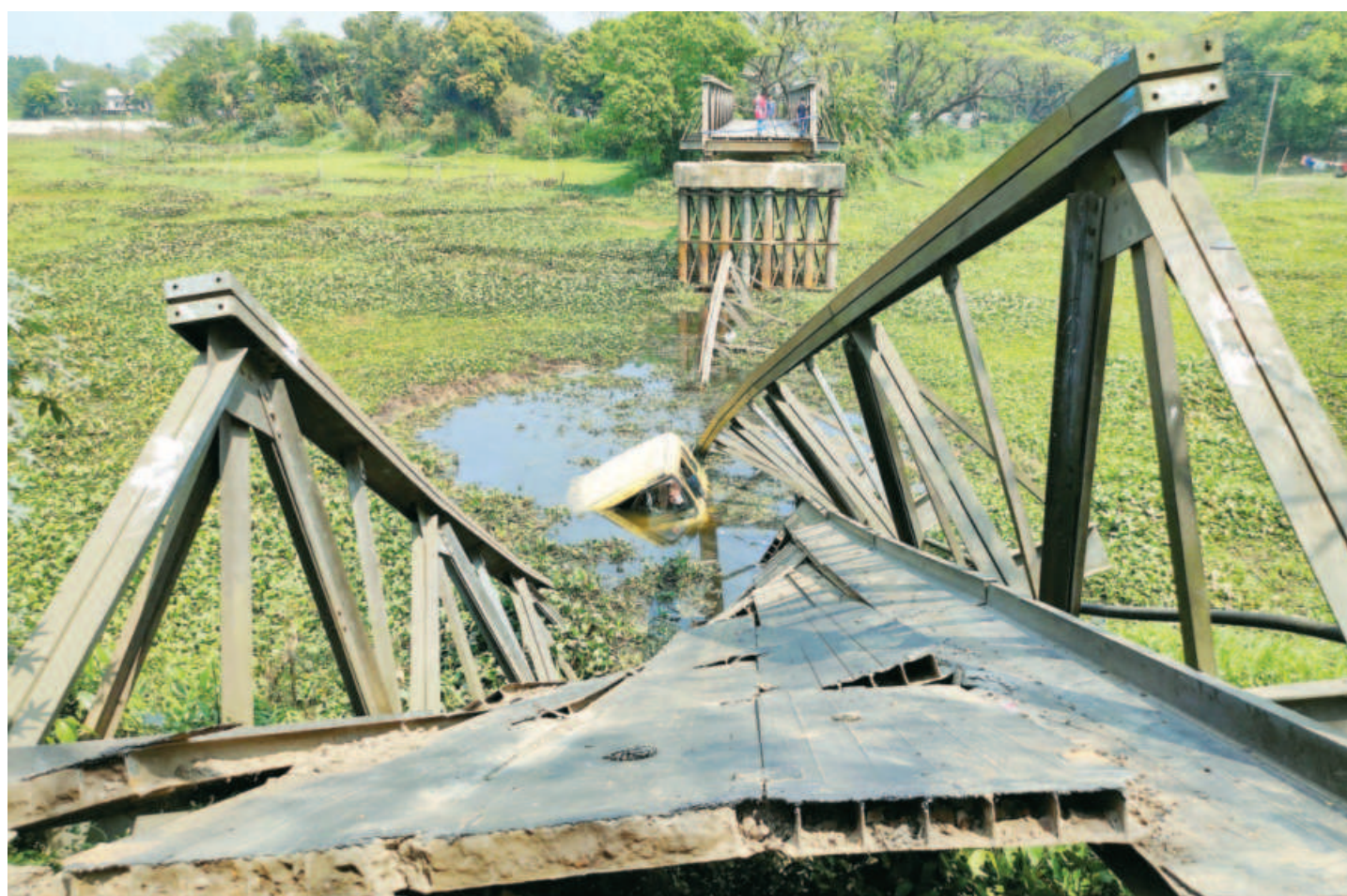
A 23-year-old Bailey Bridge collapsed in Munshiganj's Gholtoli area when a loaded truck was crossing it. The incident disrupted road communication between Tongibari and Lauhajang upazilas. Story on page 5.
