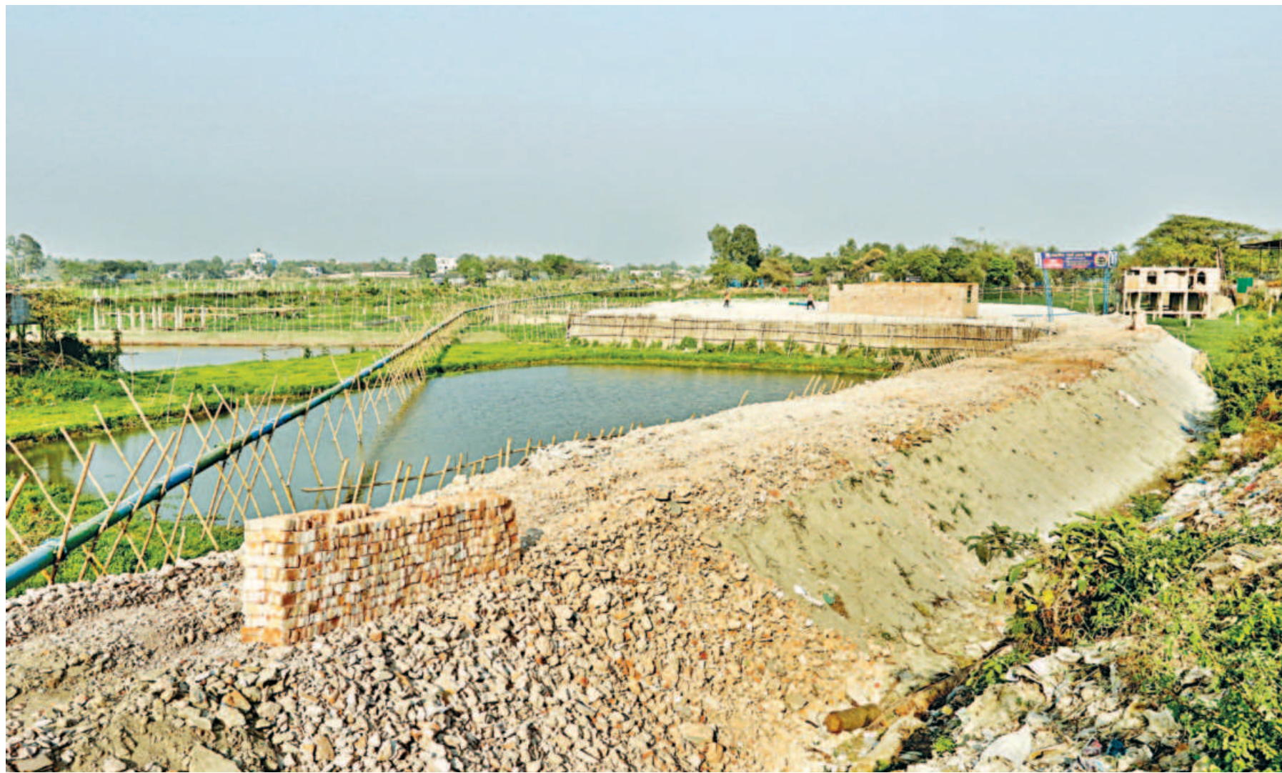
An approach road to a recreational site is being built in Nagdarpar Bazar area in the capital's Banasree. Those building the site have already filled up a portion of a flood zone to construct the road, causing environmental damage.
