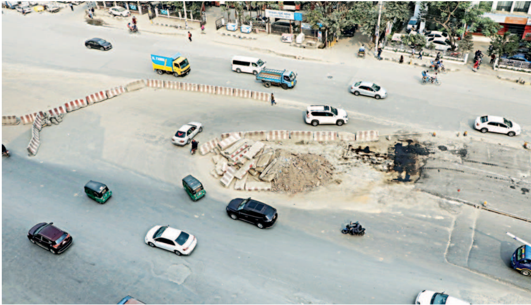
After visiting the two spots, it was seen that the U-loop near Jashimuddin Road was completely demolished, while a major part of the one in front of Rajlakshmi Shopping Complex was torn down. This photo was taken recently.
