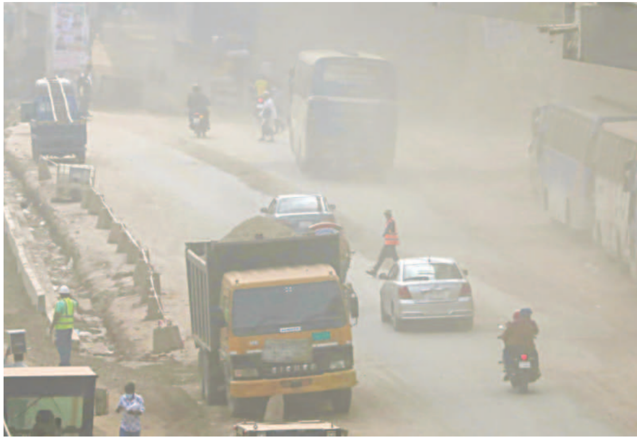
A blanket of dust covers the Tongi Bazar bus stop area in Gazipur as part of the Dhaka-Mymensingh highway is dug up for implementing a development project. The photo was taken recently.
